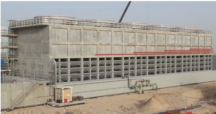
SEA WATER COOLING TOWER ROLLING MILL Project MA'ADEN, Ras Al Khair, Kingdom of Saudi Arabia
