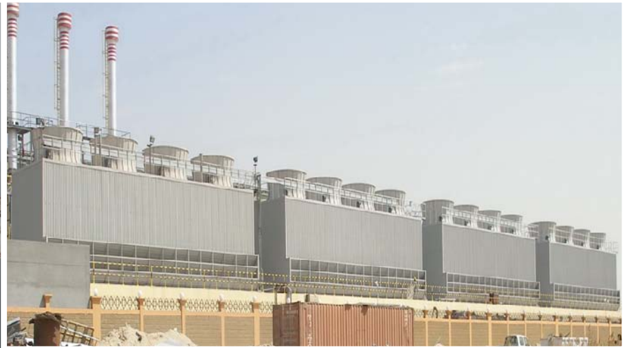
POWER PLANT, AL-Tuwairqi Steel Mill Company, Kingdom of Saudi Arabia
