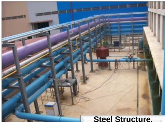
Steel Structure, Pipe Rack & Piping
