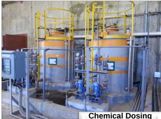
Chemical Dosing Unit
